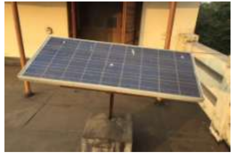
Roof-top Solar panel
